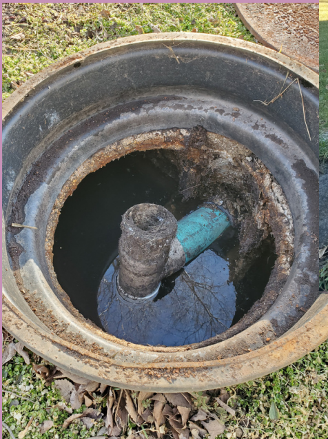
Septic tank outlet baffle showing signs of back up
